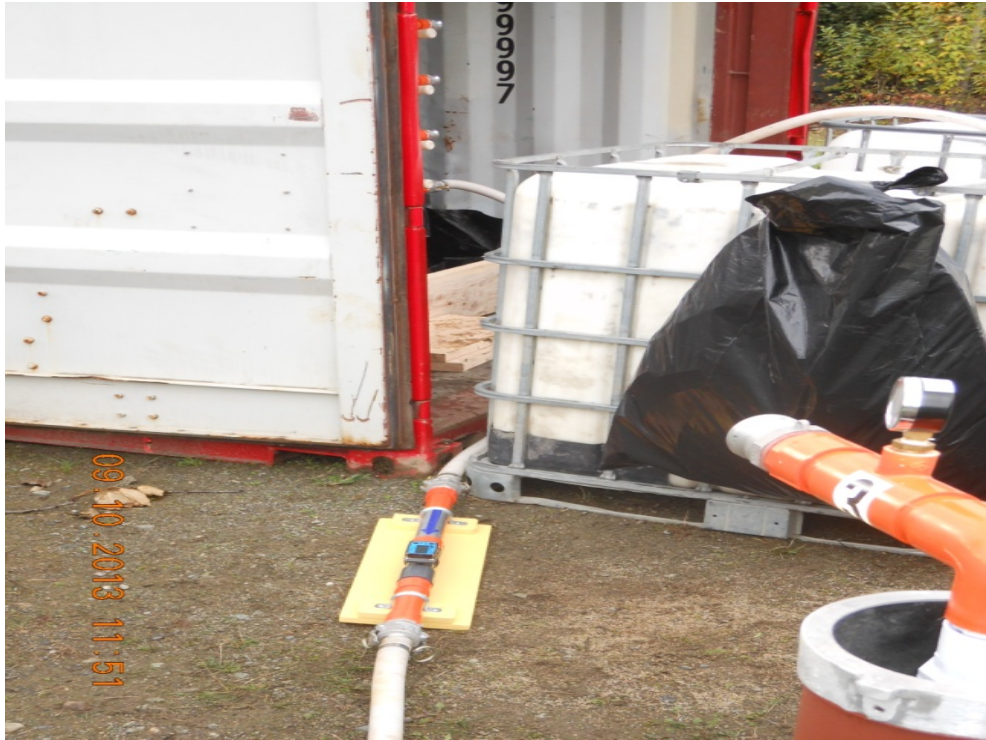
Photograph A-17: In-line totalizing flow meter (September 2013)
