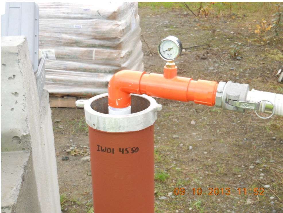
Photograph A-18: Injection wellhead assembly set up at IW01-4550 (September 2013)
