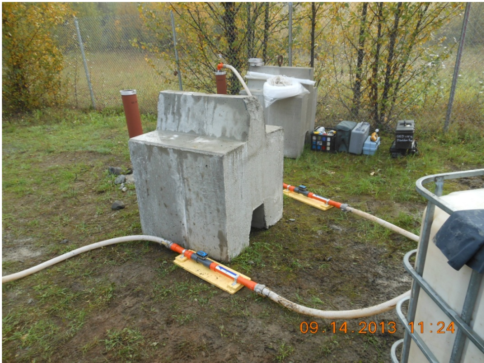
Photograph A-28: Totalizing flow meters (September 2013)
