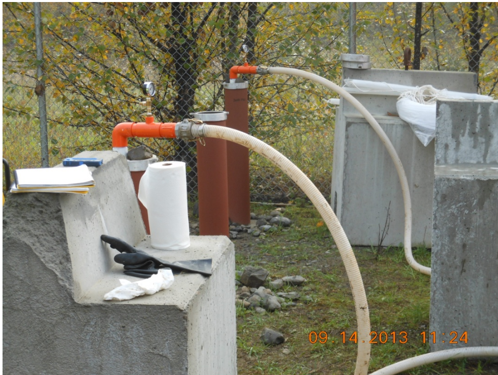
Photograph A-26: Wellhead injection assembly at AP-3983 (September 2013)
