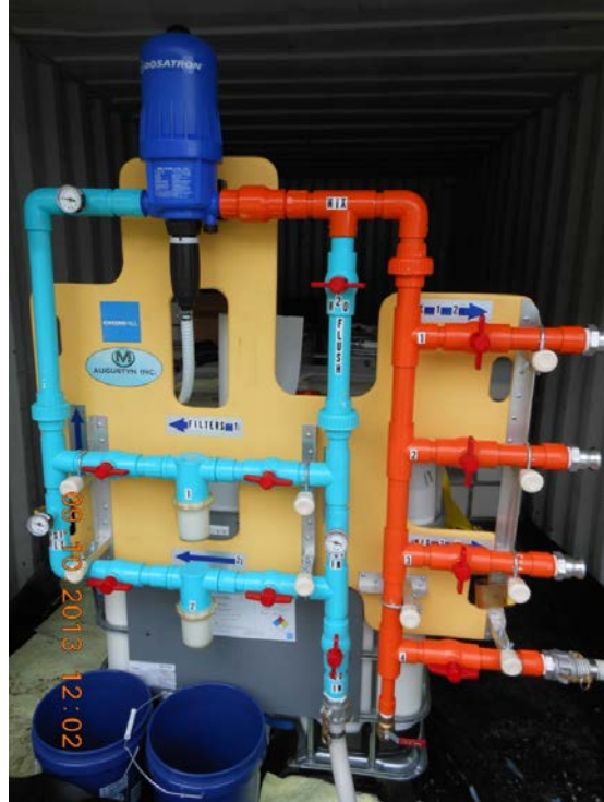
Photograph A-19: Injection system with Dosatron mounted on EVO tote (September 2013)
