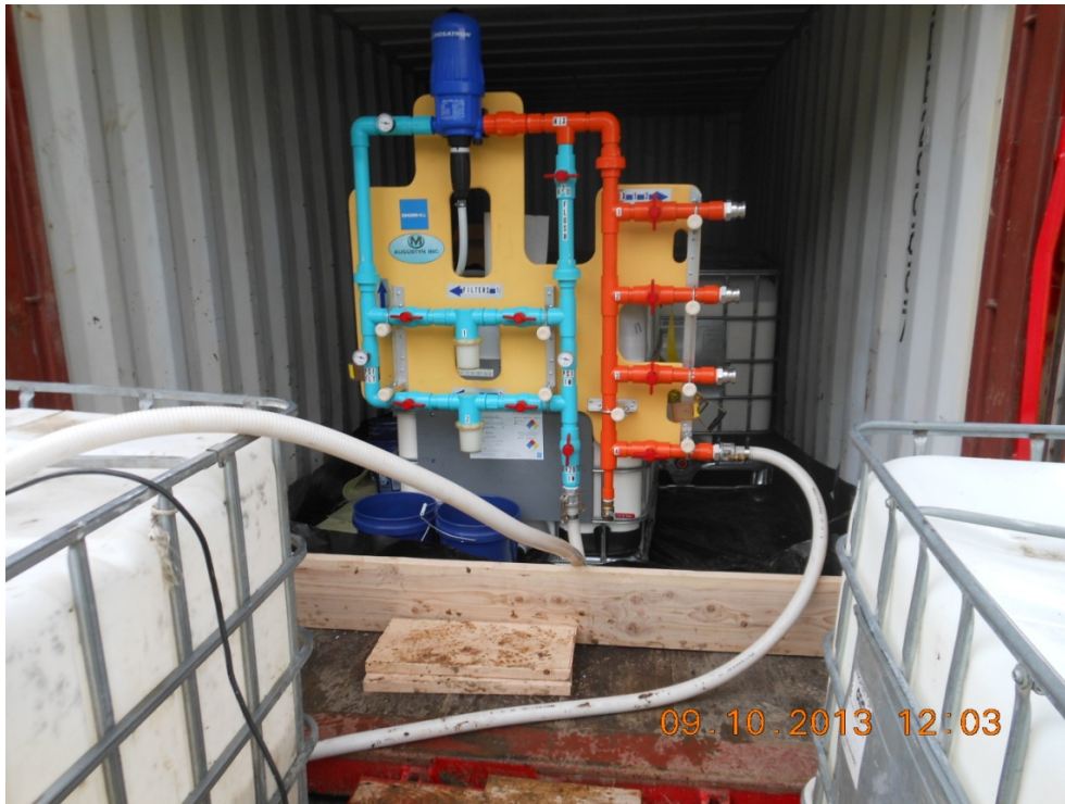
Photograph A-20: Injection system with Dosatron mounted on EVO tote (September 2013)
