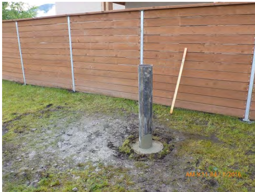
Photo A4-2: Location FS4-01; Above ground well completion
