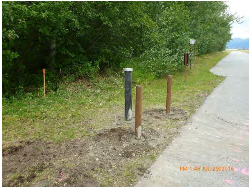
Photo A4-10: Location CHD-01; Above ground surface completion with bollards
