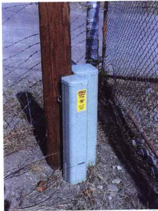
04/29/2003 – Phone Terminal Box Northwest Side of Building 986
