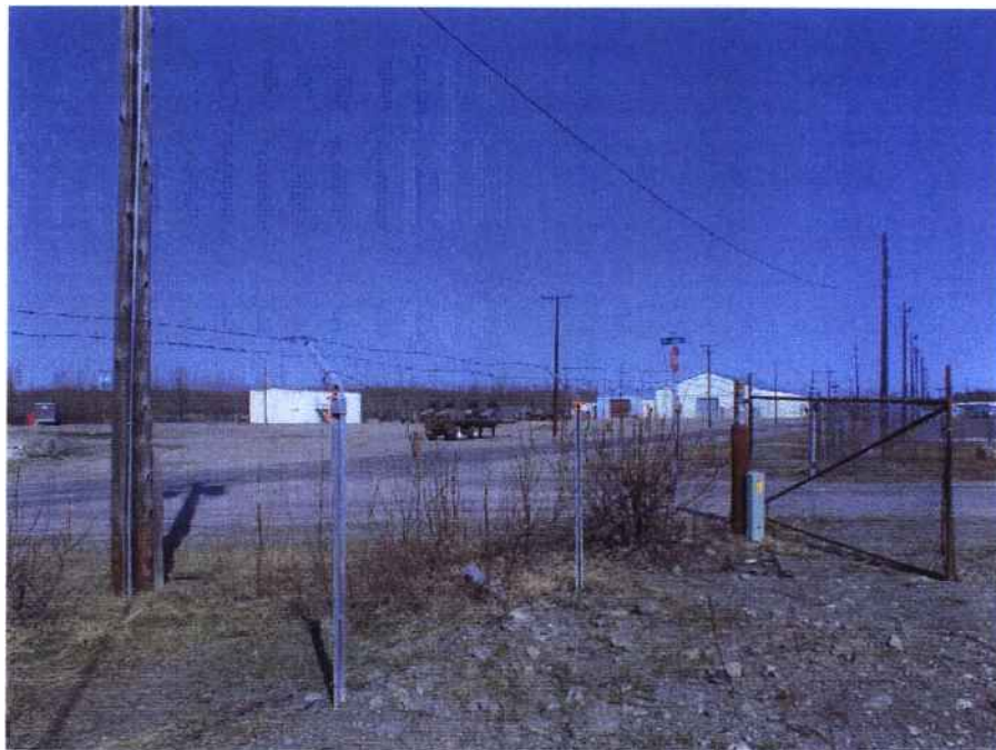
04/29/2003 – Site Electrical, Power Pole and Phone Terminal Box Northwest Side of Building 986
