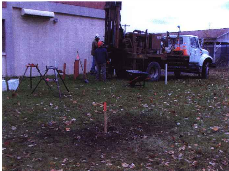
10/07/2003 – CB-13 in Foreground and Soil Boring of CB-14 South- Southeast Corner of Building 986
