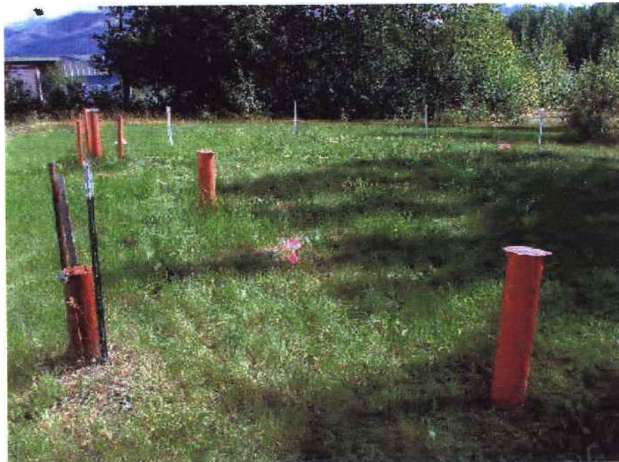
08/22/2003 – CB-13 Location and Vapor Extraction System South Side of Building 986
