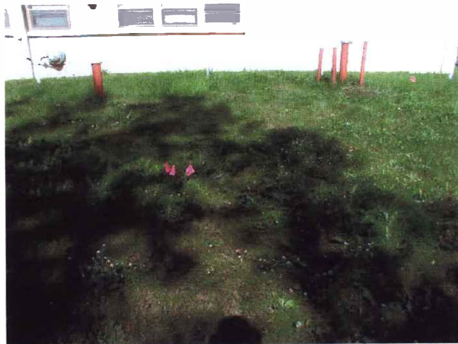
08/22/2003 – CB-15 Location and Vapor Extraction System South Side of Building 986
