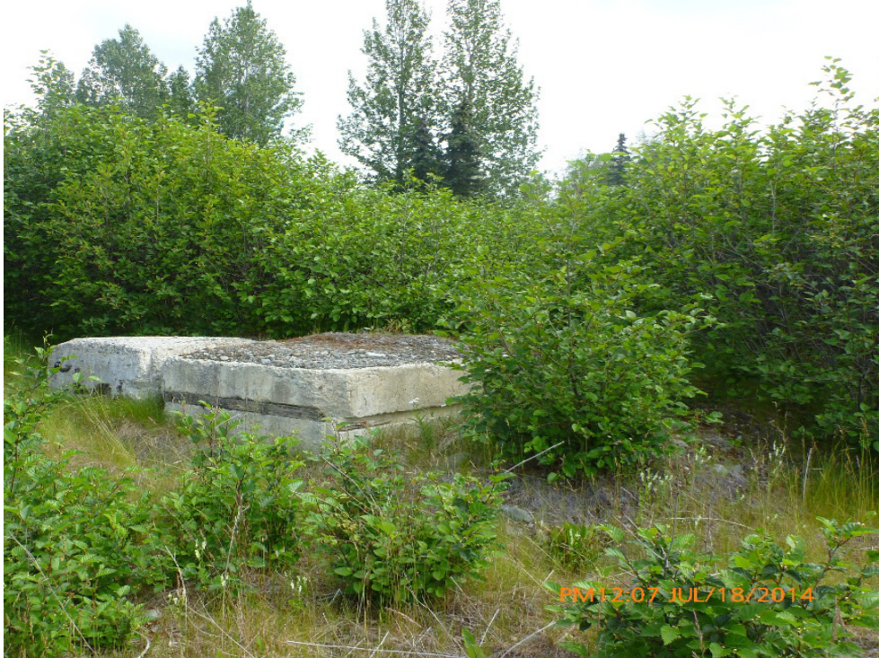
Photograph A5-15: Exposed SW corner of transmitter annex pad; densely wooded area, no other concrete exposed (July 2014).
