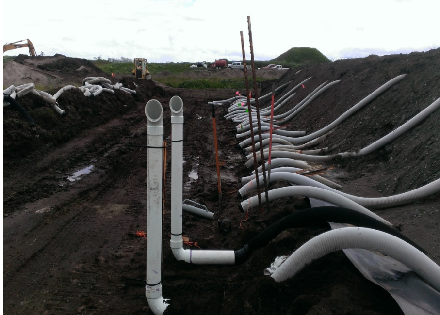
Photo No. 9 – 09 July 2014 Inlet pipes on Biopile BSB. Facing East.
