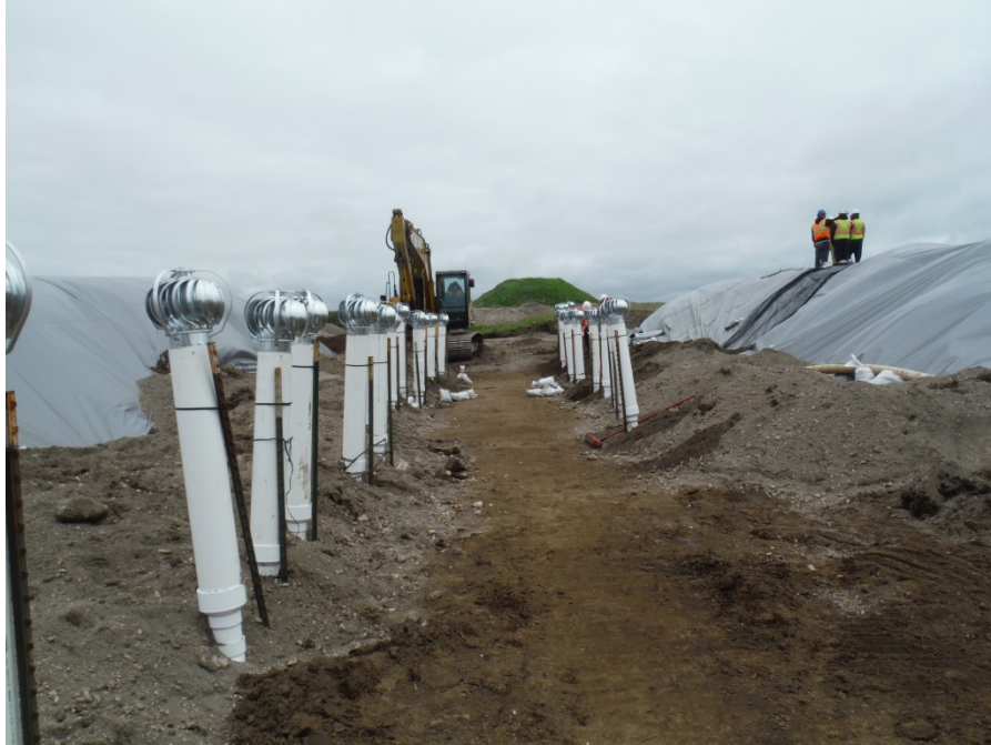
Photo No. 13 – 19 July 2014 Inlet piping on Biopiles BSA (left) and BSB (right). Facing west.
