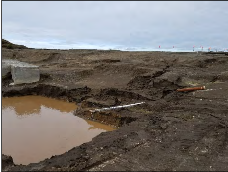
Photograph 1. Monitoring well PG-1. In 2016, another contractor excavated PCB contaminated soil from around the well. The steel casing was removed and the pvc casing was left with approximately 8 feet sticking up above the ground supported by a wood plank. In 2017 the pvc casing had broken off. View to the north-northeast. September 27, 2017.
