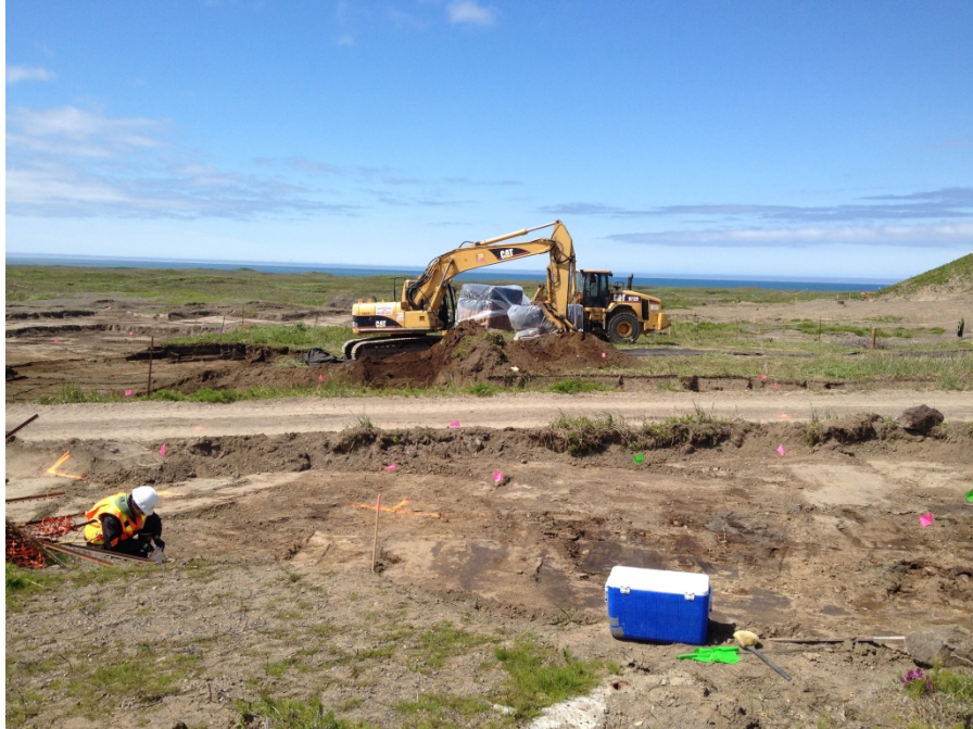
Photo No. 25 – 24 June 2014
