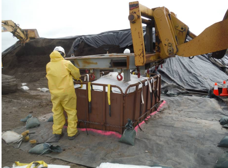
Photo No. 3 – 09 May 2014 Hooking Super Sacks to load rack. View facing south.
