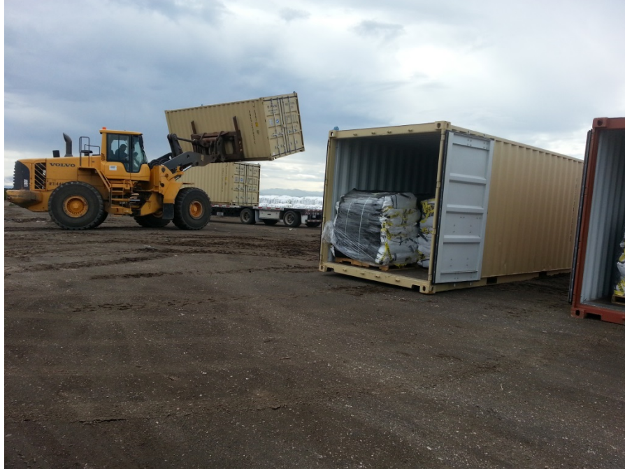
Photo No. 37 – 07 September 2014 Moving containers with Super Sacks to Storage Area J 1. View facing southeast.
