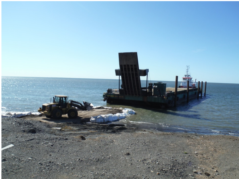
Photo No. 32 – 31 August 2014 KEMRON and ELM Solutions constructing the barge landing ramp. View facing west.
