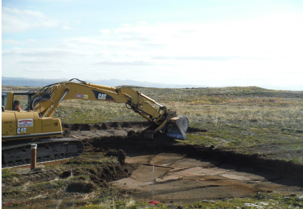
Photo No. 45 – 29 September 2014 Excavating non-TSCA soil in Soil Removal Area 2. View facing southwest.
