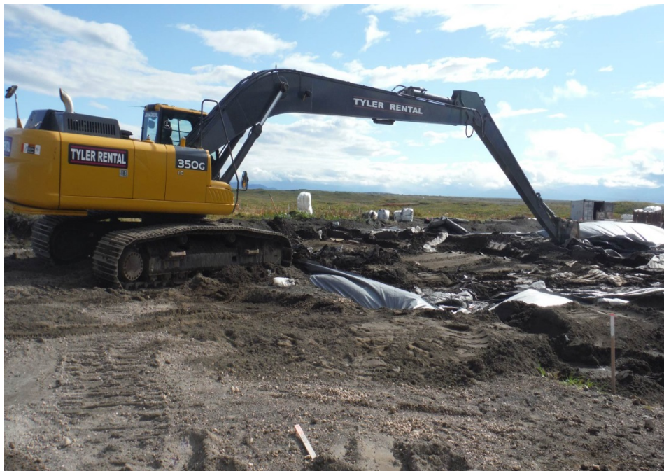
Photo No. 40 – 16 September 2014 Excavating non-TSCA PCB soil from stockpile CA 4. View facing south.
