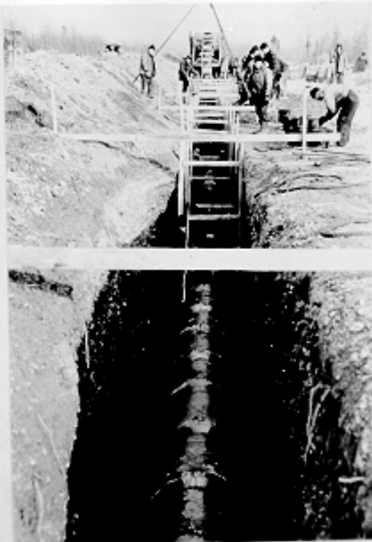
Looking east from a point approximately 1 mile west of Fort Richardson, showing construction of Gravity Sewer Line. 3-13-41
