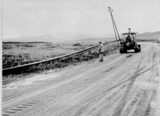
Welded section of pipe line being transported to loca- tion near Satellite field. Nome Garrison Project, Alaska. 9-26-42
