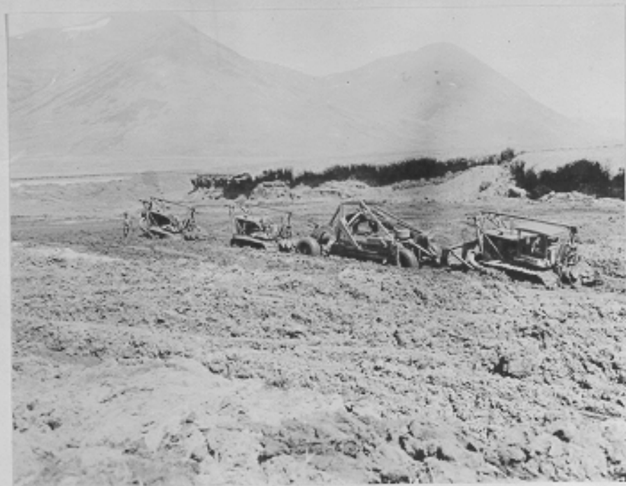
(C496C) Typical example of difficulty encountered in stripping muskeg. 3 cats required to load 1 carryall. Runway "A", Alexai Point, Attu Island, Alaska. 6-17-43
