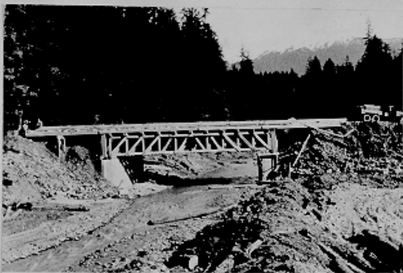
Bridge over North Creek built by 331st Engineers, looking east. Excursion Inlet, Alaska. 4-26-43
