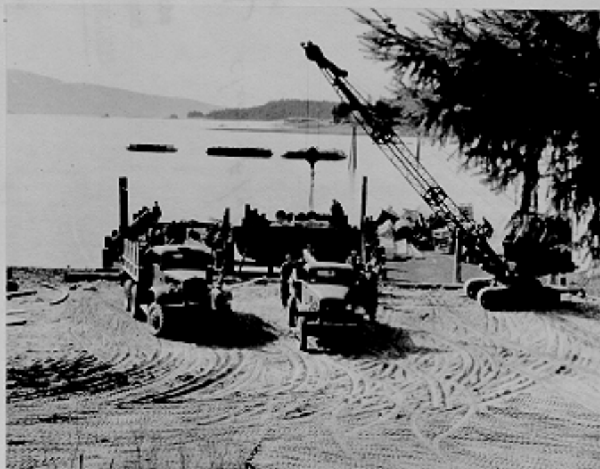
Unloading construction materials from barges (C498B) at Auke Bay. CAA Garrison, Juneau, Alaska. 4-23-42
