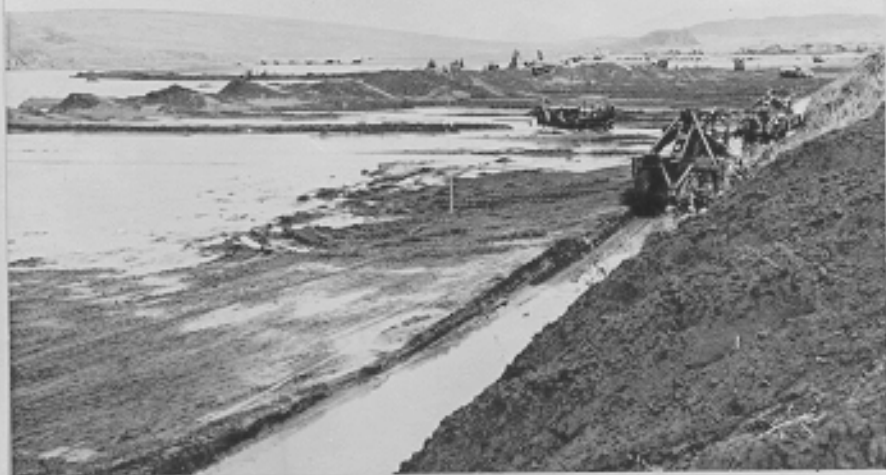
Looking north on southern extension of "A" runway. Present field within dike, upper left. Adak, Alaska. 9-1-42
