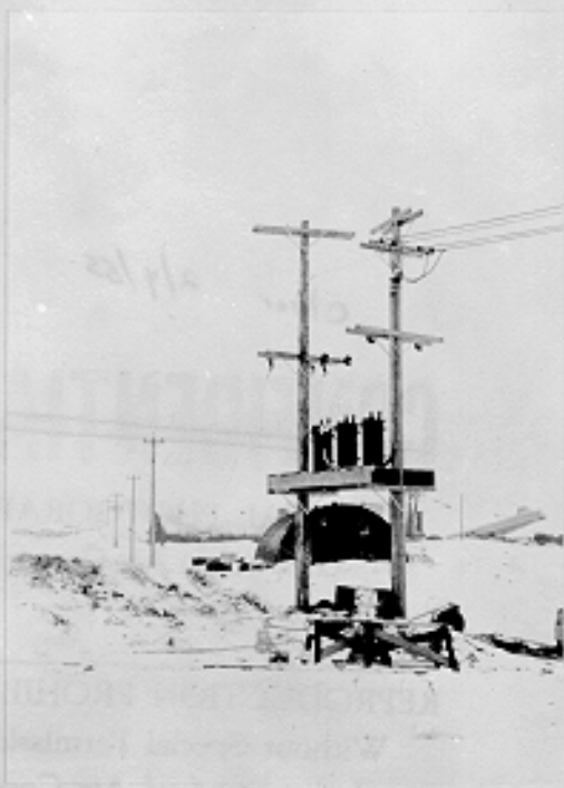
Transformer bank near laundry from road looking east. Nome Garrison Project, Alaska. 12-1-42
