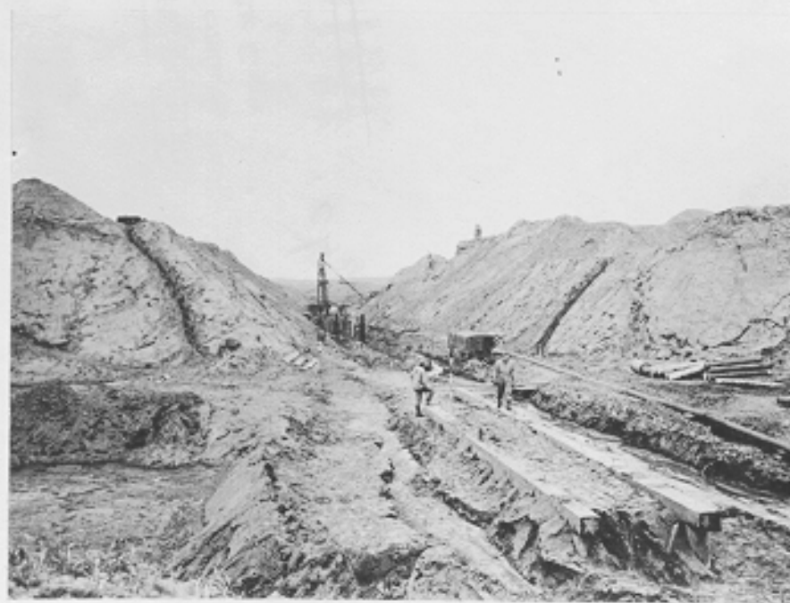
(C496B) Runway construction showing fill and culvert Station #0" (washout area). Shemya Island, Alaska. 7-7-43
