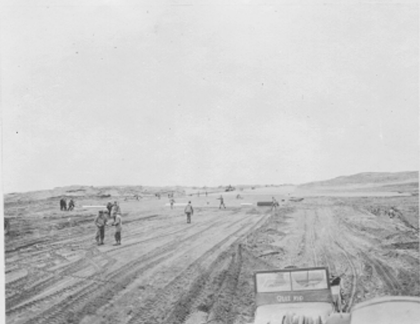
Runway construction showing portion completed steel mat. Looking west from Station "O". Shemya Island, Alaska. 7-7-43
