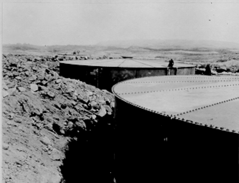
Gas storage tanks ready for camouflage. Amchitka, Alaska. 5-19-43
