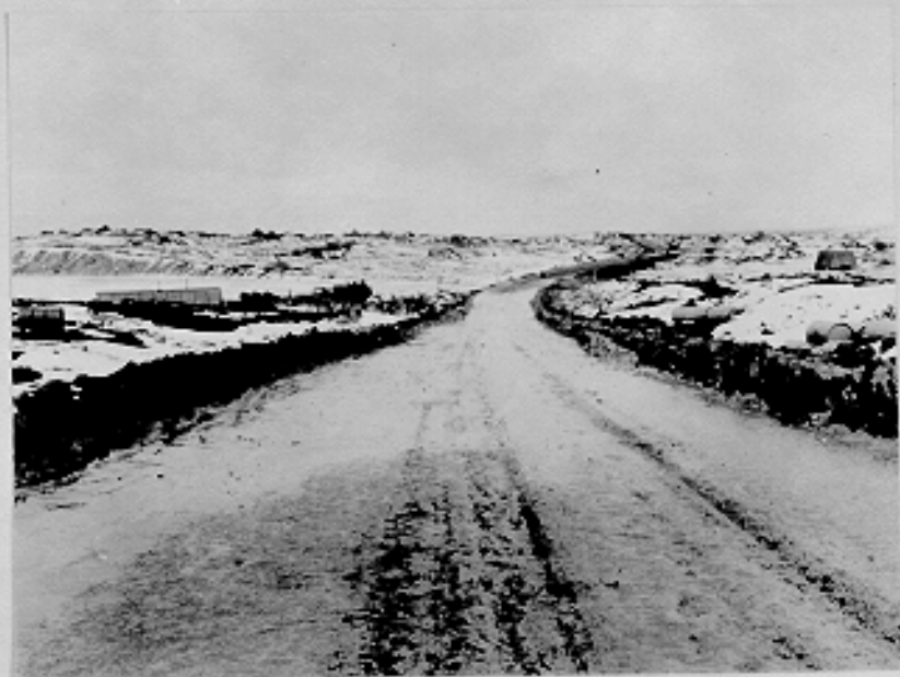
Umanak Island - Construction road between gravel pit and runways. Fort Glenn, Alaska. 7-7-42
