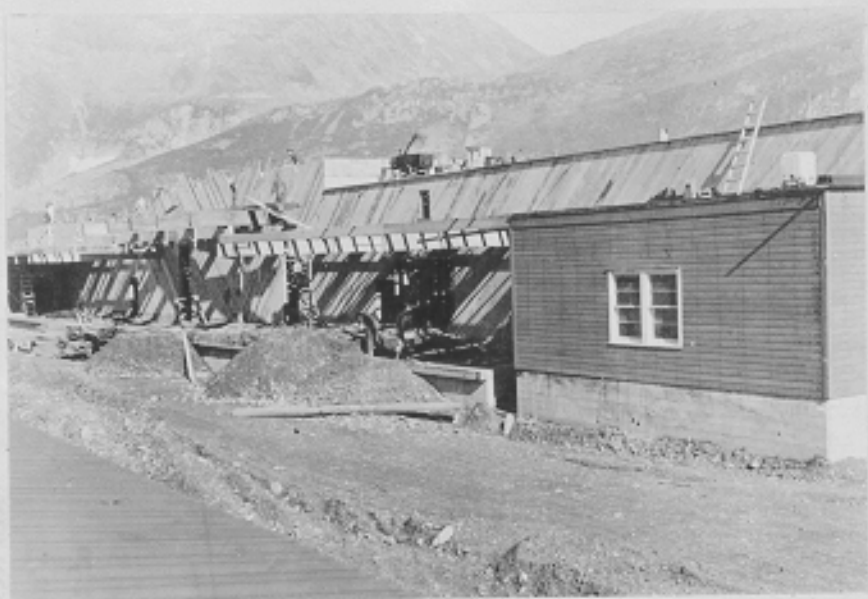
Refrigeration plant from the top of a boxcar in the railroad. Note cantilever beams at front canopy. Alaska Railroad Passage Canal, Whittier, Alaska. 8-1-43
