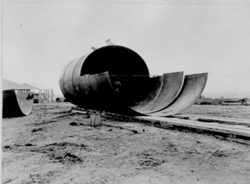
Gasoline tanks being put together with welding shed in background. Fort Glenn, Umanak, Alaska. 6-10-43
