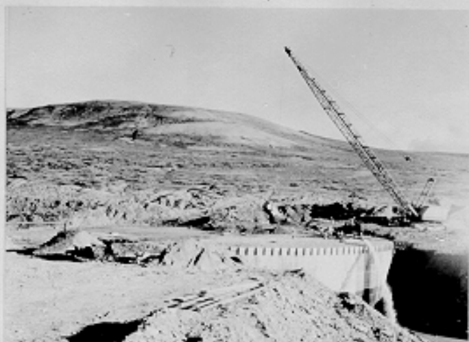
Test water flowing from tank #1, gasoline storage shovel and dozer backfilling. Nome Garrison Project, Alaska. 10-5-42
