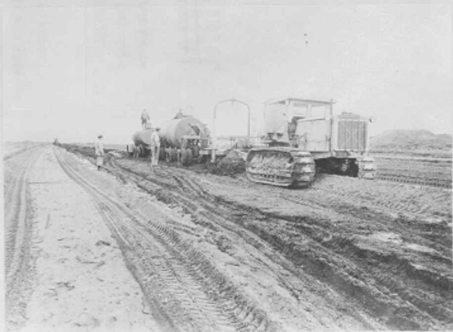
(C496G) East-west runway. Pouring Bitumin on North half. Cold Bay, Fort Randall, Alaska. 8-4-42
