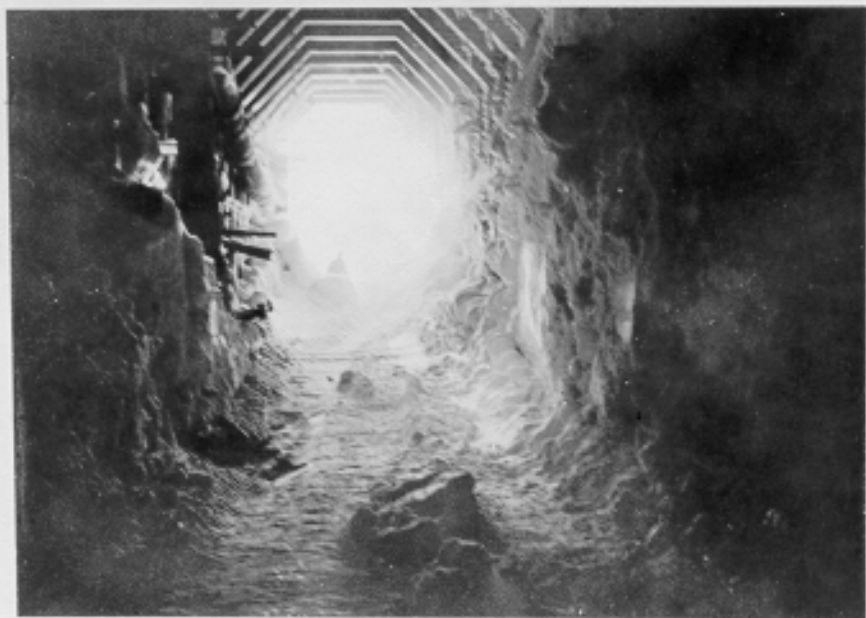
(C508A) Drifted snow at entrance to snowshed also heavy frost formed by condensed tunnel vapor. Picture taken from portal, set looking south. Alaska Railroad Cut-Off Project, Whittier, Alaska. 1-10-43
