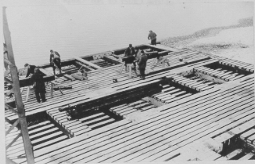
(C503A) MNAF - Seaplane Ramp, decking in place and openings for counterweight blocks shown in flooring. Yakutat Landing Field, Alaska. 1-20-43
