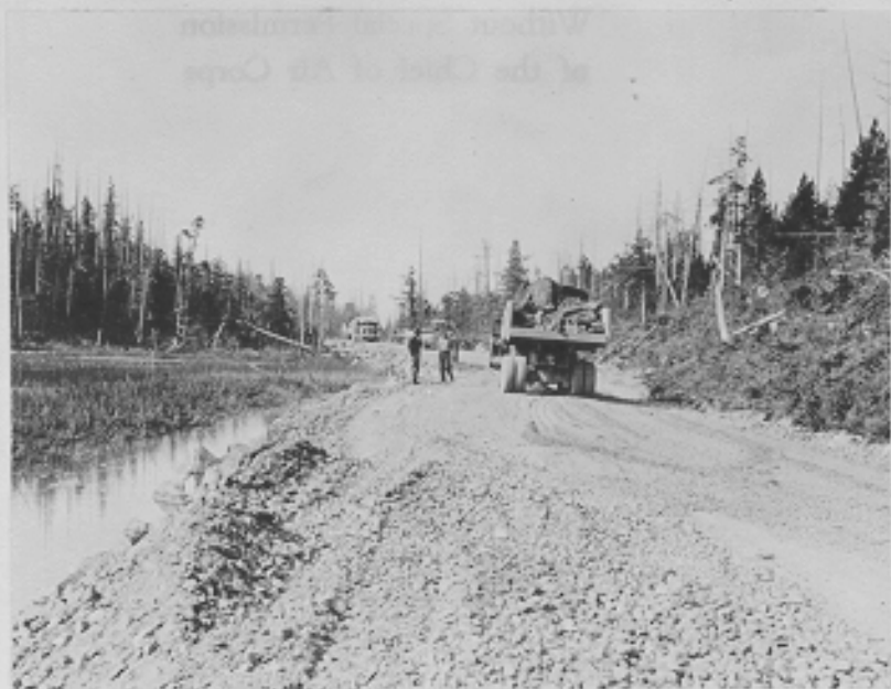
Rock fill on the Metlakatla road. Notice to the left that the mud and sand is being pushed up from the ponds. Looking west from station 48+00. Annette Island Landing Field, Alaska. 7-31-42
