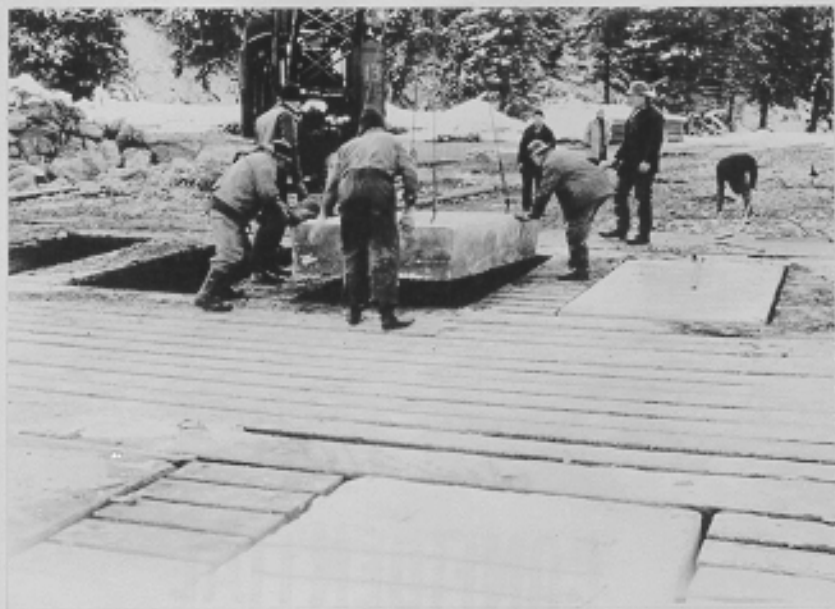
Concrete counterweight block being placed in inboard section of ramp near anchor block. Yakutat Landing Field, Alaska. 2-8-43
