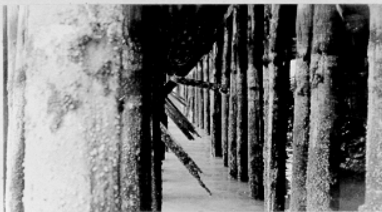
Femmer dock piling. Braces consumed by teredos. These marine boring worms have been known to com- pletely collapse entire docks of untreated piling (C513B) within four months. Juneau Sub-Port of Embarka- tion, Alaska. 7-24-42
