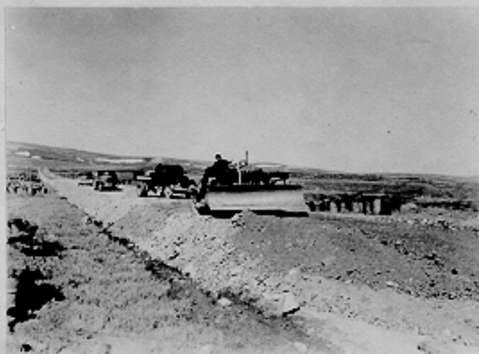
Bessie Road fill near the S & A Battery, 81st F.A. Nome Garrison, Alaska. 6-9-43
