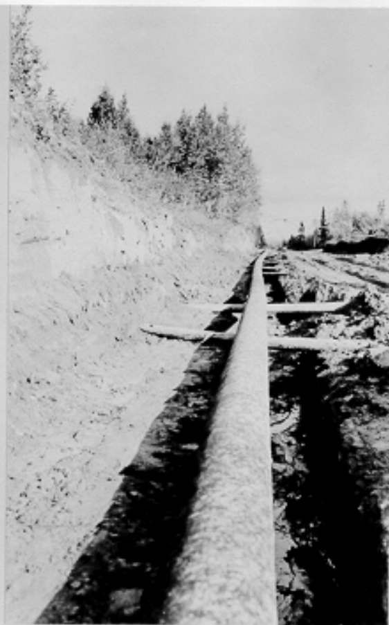
Gasoline pumping line looking toward Fort Richardson from gasoline pumping station. 10" main gas line. Fort Richardson, Alaska. 9-14-42
