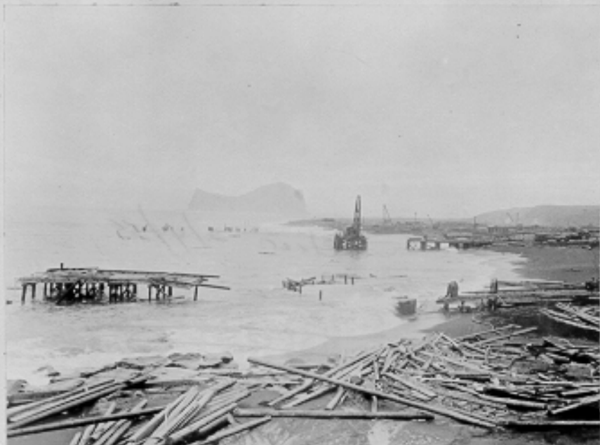
General view of barge dock damage and debris caused by storm and loose barges. South Fustoi Bay, Fort Glenn, Alaska. 9-22-42
