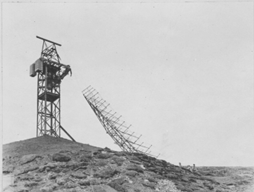
Hoisting of antenna and antenna in place on detector building. AWS Cape Prominence, Alaska. 6-15-43
