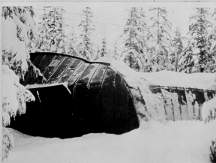
Warehouse damage, Cordova, Alaska. 1-14-43
