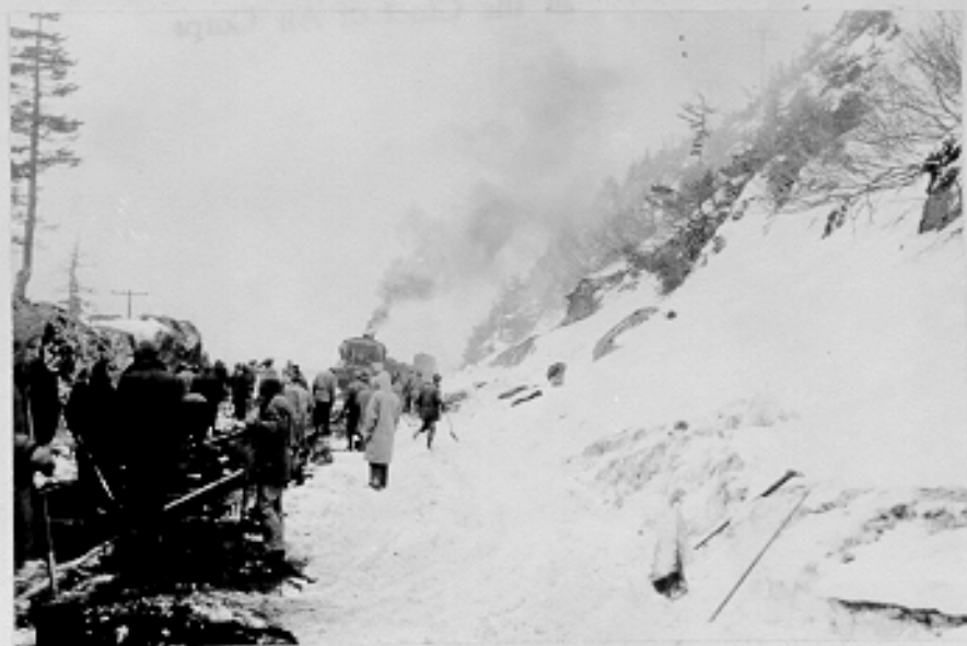
(G507) Ballast train approaching through cut at station 57 + 00. Ballast crew in foreground. Alaska Railroad out-off Project, Whittier, Alaska. 4-5-43
