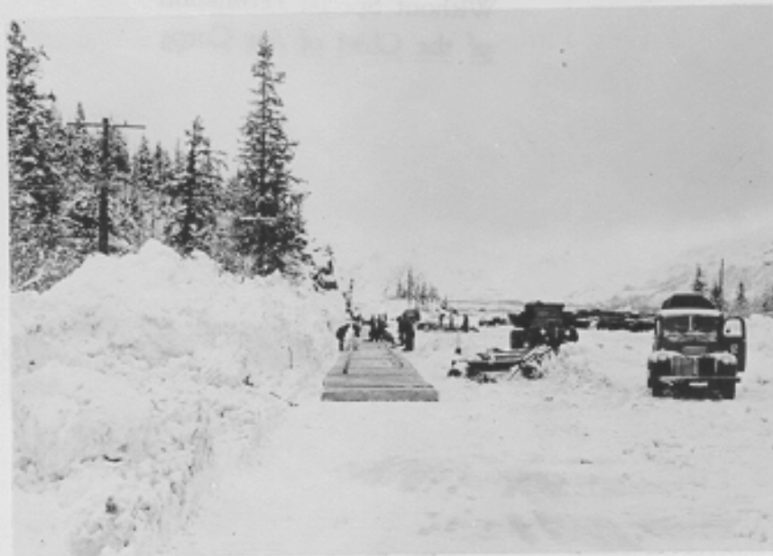
(C507C) Laying track in Railroad yards. Note snowbanks of dozed snow. Accumulative snowfall this date about 8'. Alaska Railroad Cut-Off Project, Whittier, Alaska. 2-2-43
