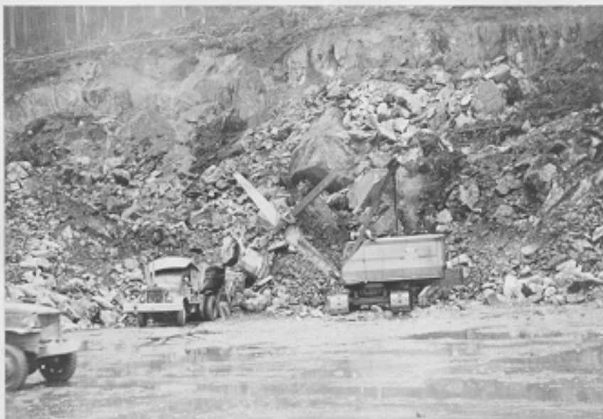
Hauling muck away from quarry face after shooting two coyote holes, looking east. Excursion Inlet, Alaska. 2-23-43
