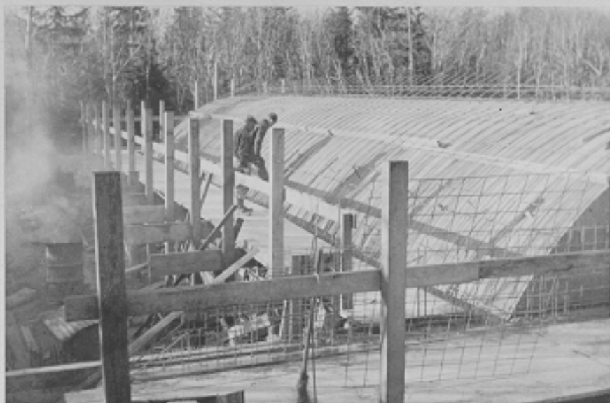
(C505) Concrete underground magazine after first lift of 6' was poured. Salamanders were required to keep concrete from freezing. Chilkoot Barracks, Alaska. 11-4-42
