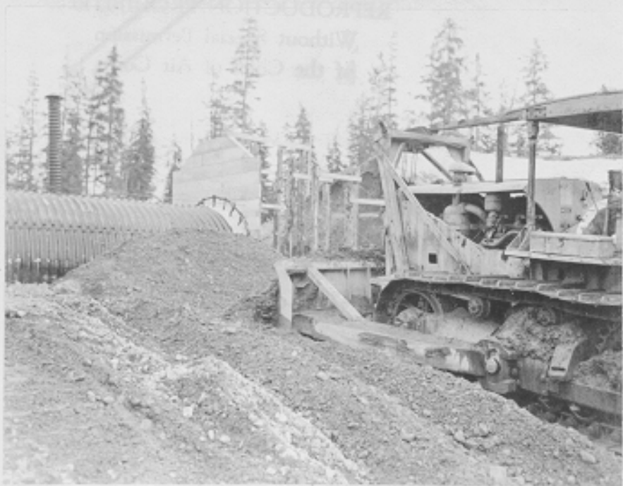
Backfilling elephant shelter ammunition storage (C505A) (using a D-8 bulldozer). CAA Cordova, Alaska. 4-8-43
