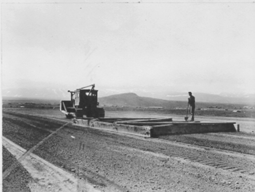
Gravel, volcanic ash, pierced steel plank or concrete -- the work was done quickly with the materials at hand to meet or better the completion dates.
