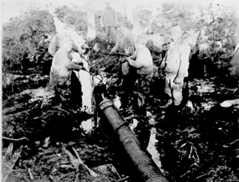
Laying wood stave pipe for Yellow Lake water line, looking north from station 80+00. Annette Island Landing Field, Alaska. 1-10-43
