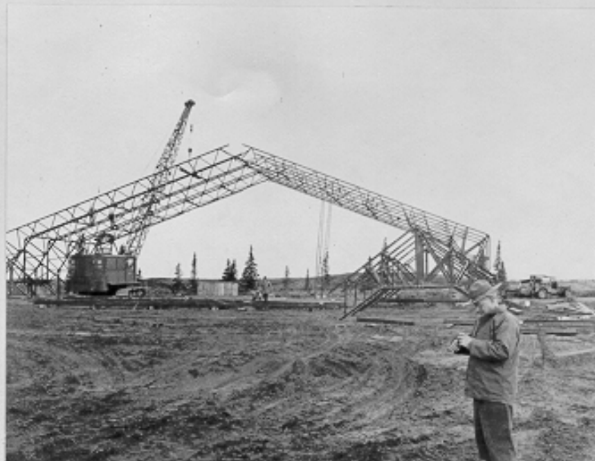
Aviation Engineers portable hangar under construction near future taxi strip. CAA Naknek, Alaska. 8-26-43
