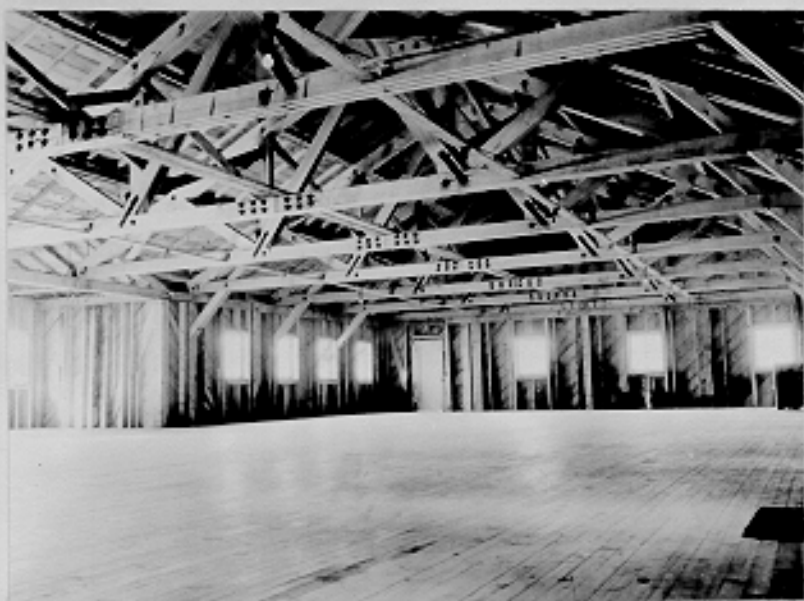
Interior view of 40' x 80' Recreation building in construction camp. CAA Garrison, Juneau, Alaska. 3-5-43
