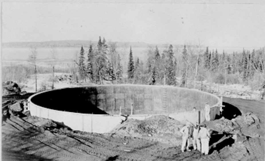
Fuel oil storage. Concrete storage tank No. 1 (10,000 barrel). Fort Richardson, Alaska. 10-11-42
