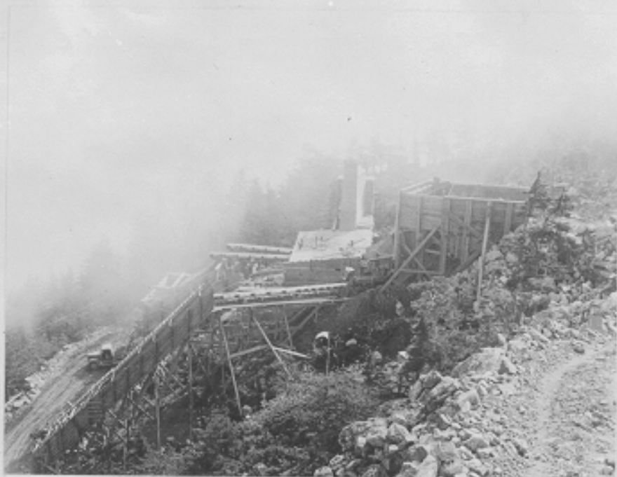
Aggregate crushing plant, Battery 294. Conveyor belt and long bin in foreground takes out fine, ahead of crusher, for road surfacing, looking east. Seward, Alaska. 8-2-43
