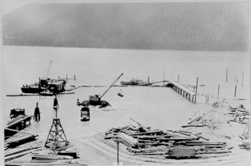
(C502 A) Dredging for Marine Ways at north end of dock unit #1, looking west. Excursion Inlet, Alaska. 8-3-43
