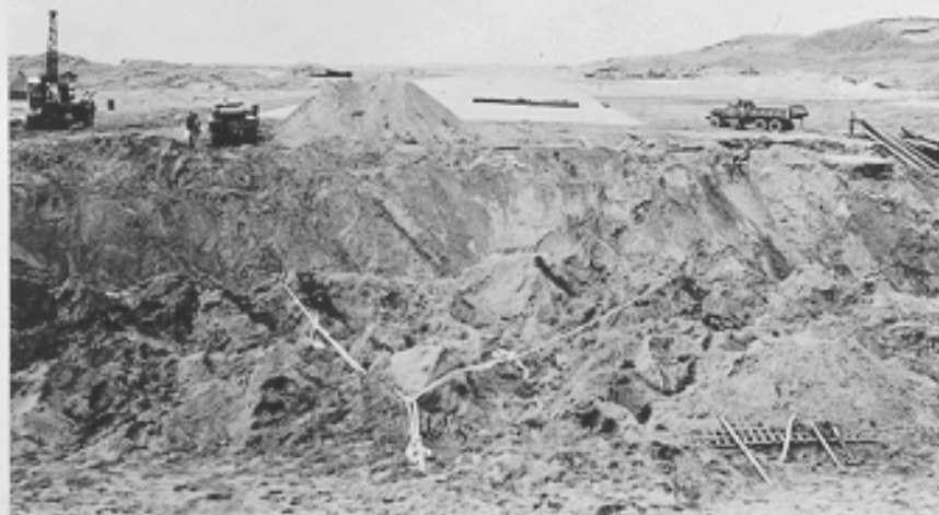
Completed portion steel mat - locking west from washout area - Shemya Island, Alaska. 7-7-43
