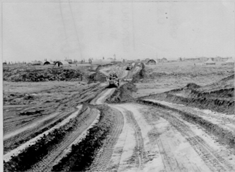
New road across Eskimo Creek from construction area to garrison area. CAA Naknek, Alaska. 8-17-43 (C492E)
