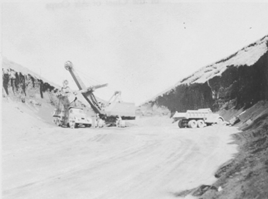
(C509B) Umnak Island - shovel and trucks loading cinder-gravel material for road and runway construction. Pit located across 33 creek from 802nd camp. Fort Glenn, Alaska. 7-7-42
