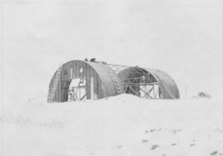
Cowin hut under construction in Satellite area - view taken from road, looking south- east. Nome Garrison, Alaska. 12-1-42
