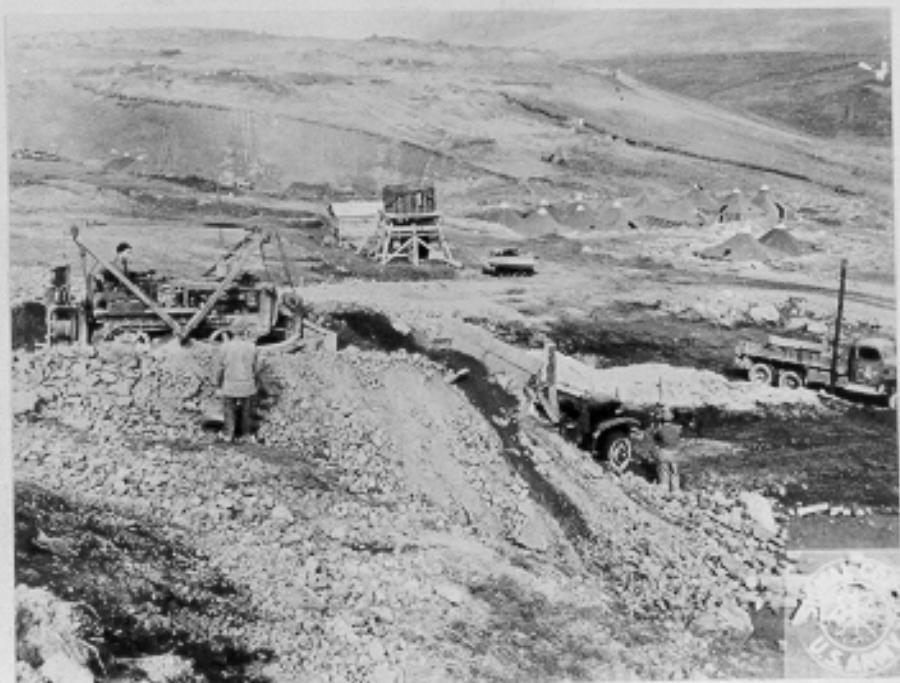
Race Hill Road Pit. View of initial stage of (C509) development using dozer loading. Kiska Island, Alaska. 9-19-43
