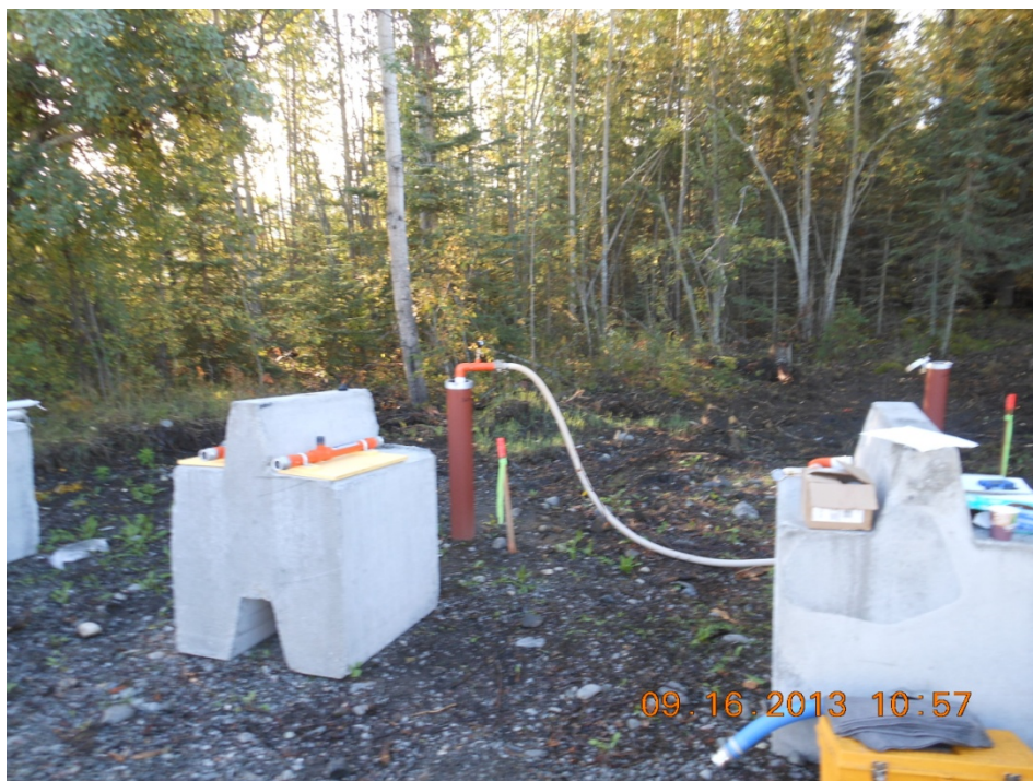
Photograph A-14: Wellhead assembly and hoses at IW04-4413 (September 2013)
