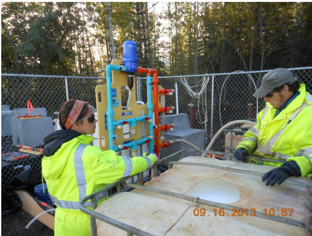
Photograph A-12: EVO batch injection mixing tank (September 2013)
