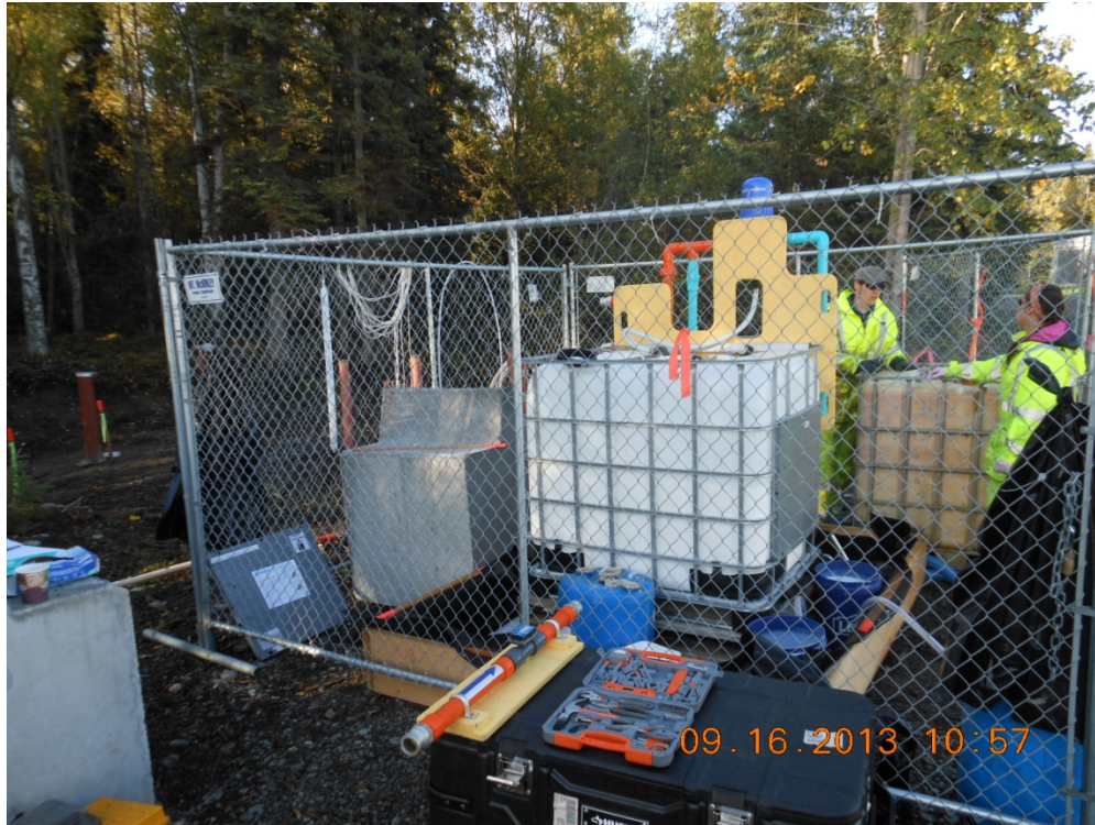
Photograph A-11: Injection system at DA085 (September 2013)
