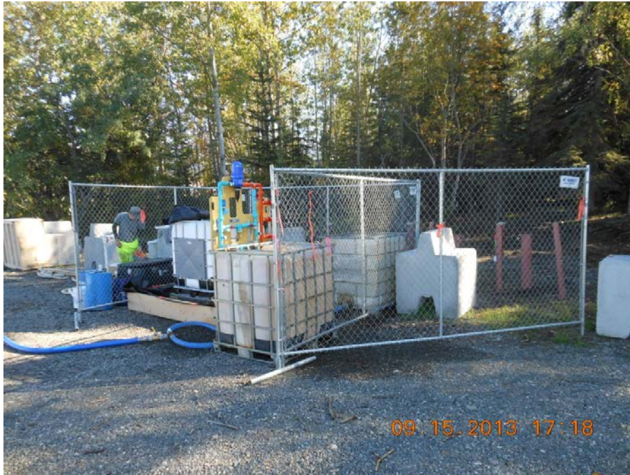
Photograph A-9: DA085-IW01-4413, injection system setup at DA085 (September 2013)
