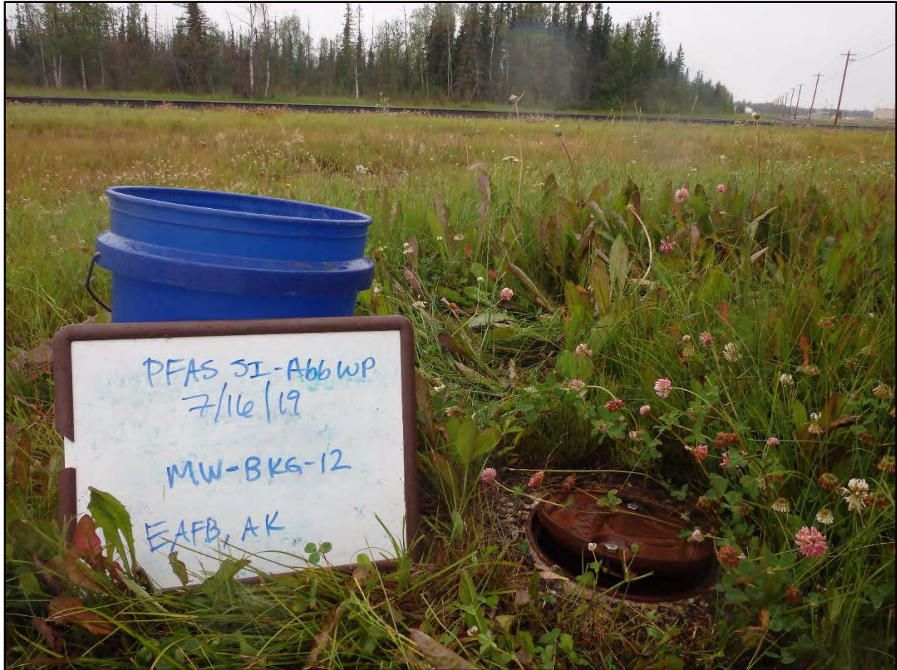
Photograph C.1-8. View of broken outer casing of MW-BKG-12.
