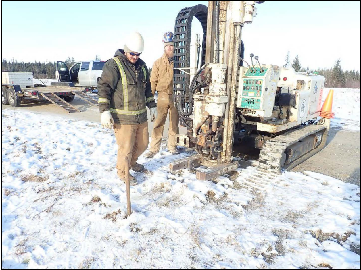
Photograph C.3-15. SP-16 temporary well ready for purging at TW03.
