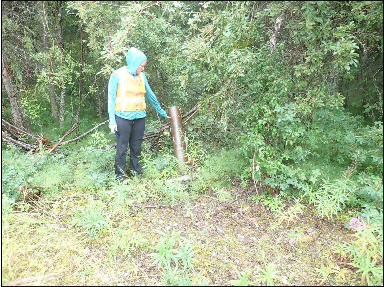
Photograph C.1-4. View of 51MB4 damage.
