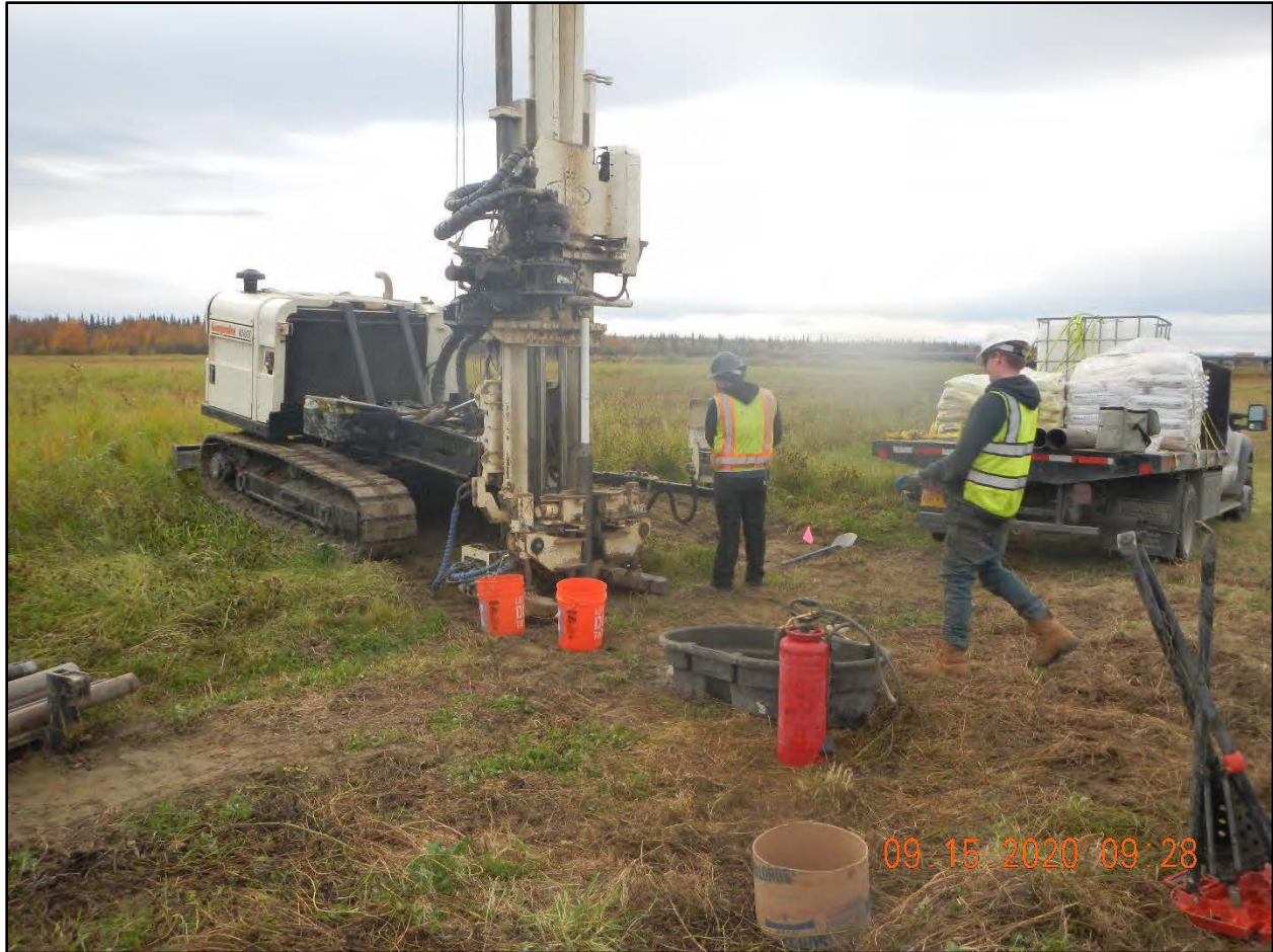
Photograph C.4-6. Previous drill location for MW-23 where refusal was encountered and new drill location offset 15 feet.
