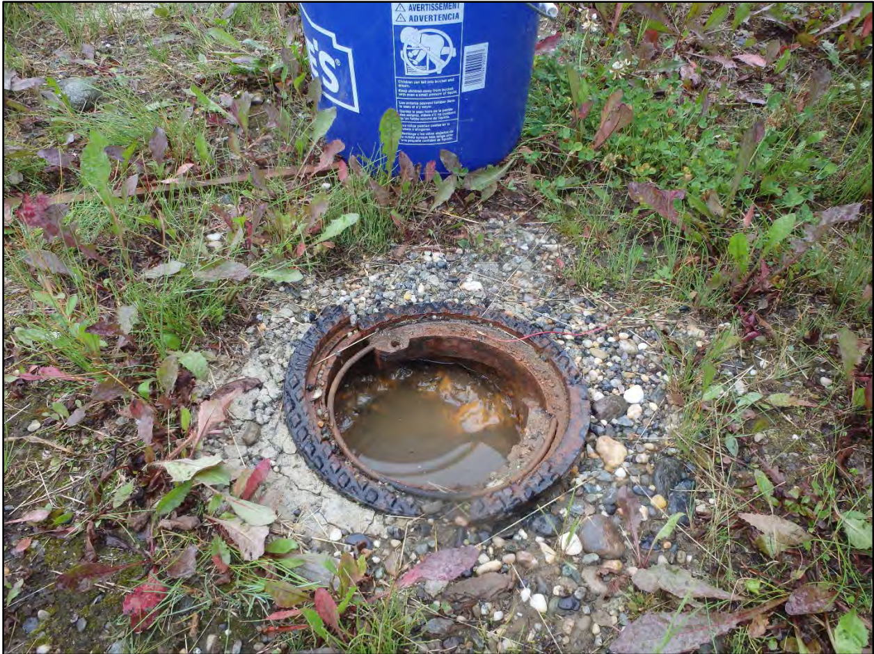
Photograph C.1-7. View of broken outer casing of MW-BKG-05.
