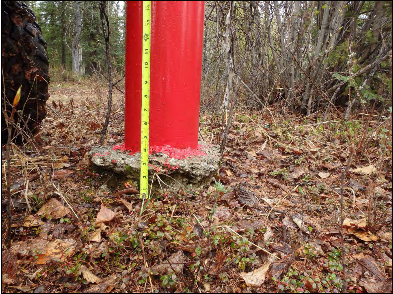
Photograph C.1-16. View of frost jacking of USAP-3.
