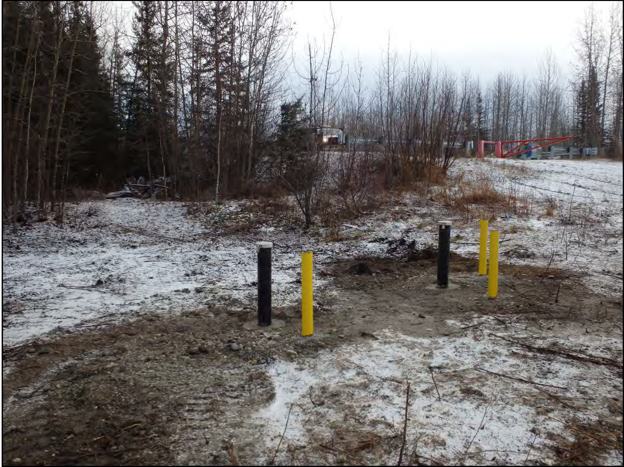
Photograph C.2-13. View of completed wells 19PS-MW1A and 19PS-MW1B and bollards in Well Cluster #1 area.
