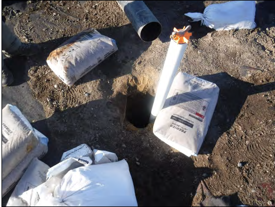
Photograph 75: Cavity observed at MW-10 during attempted well development. Cavity observed to extend approximately 24 feet below ground surface (ft bgs). 29 Jul 2018.
