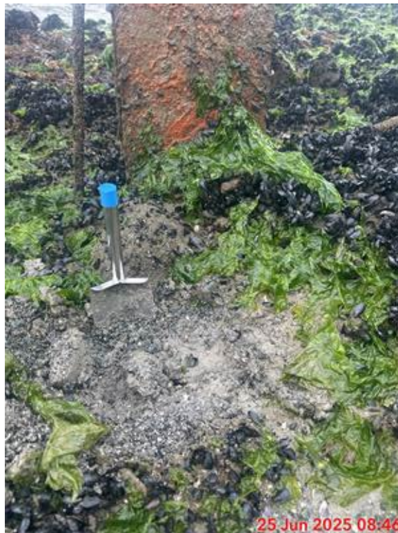
Photograph 42: Sediment at 6 inches deep at leg of South Dolphin. View East. 6/25/2025.
