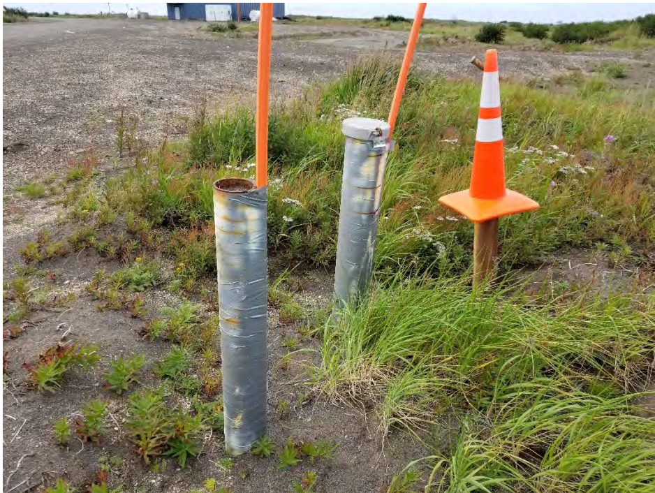
SS006 (FPC-215) - Monitoring Well MW-9 is secure and in good working condition.
