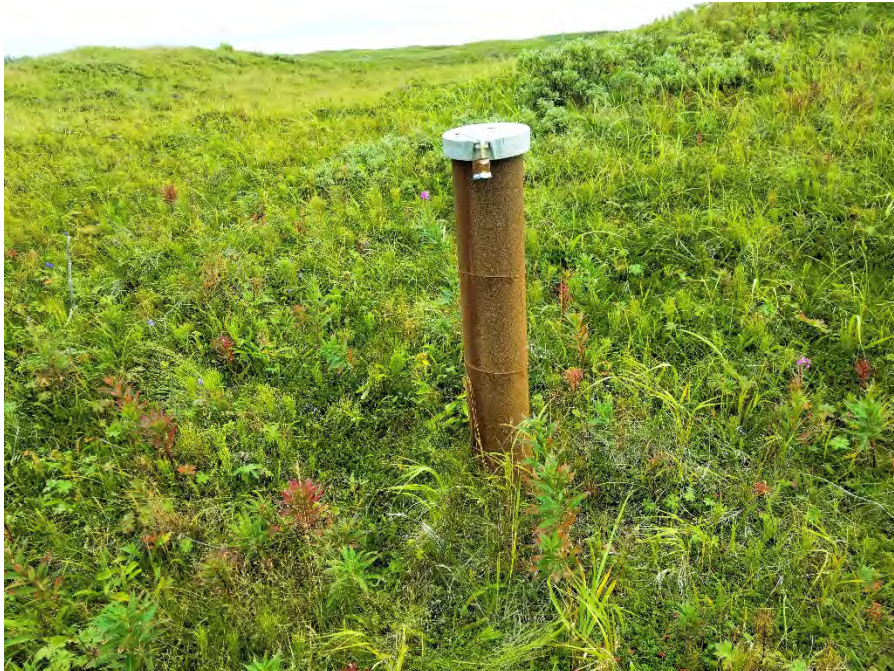
WP002 - Monitoring Well BLO-MW-02 is secure and in good working condition.
