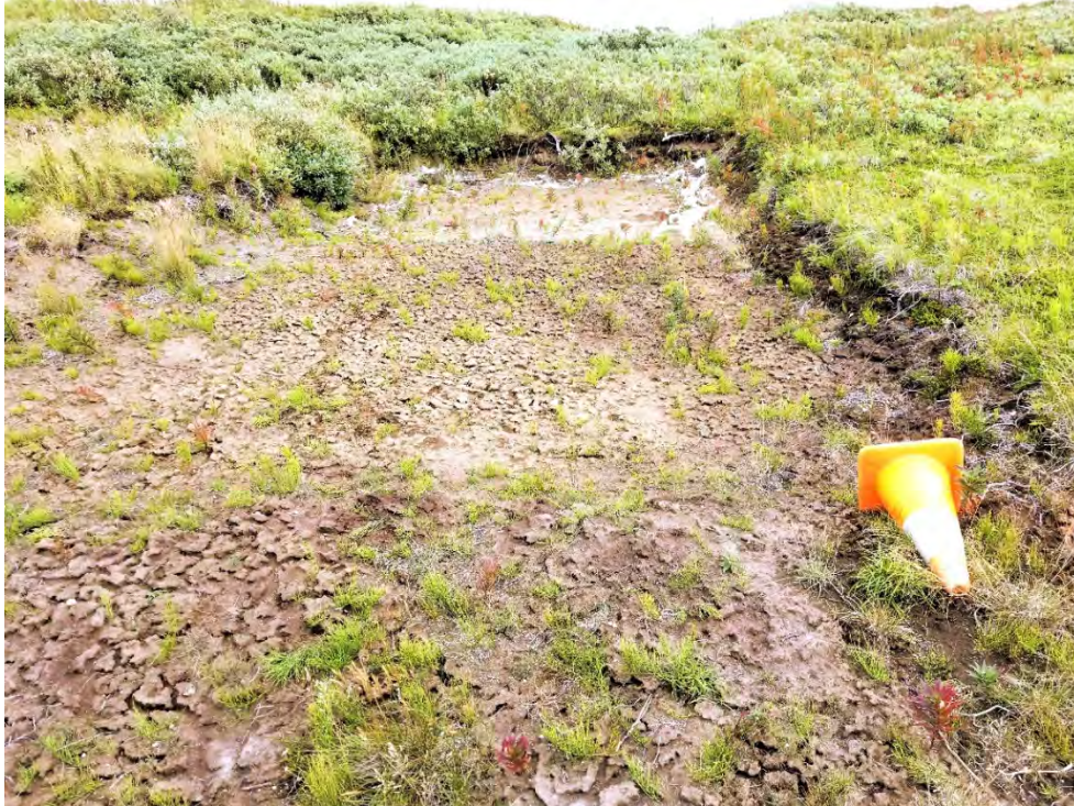
SS004 – Septic System Outfall, a view of what remains at the outfall.
