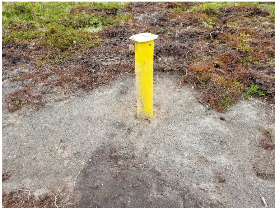
LF007 - Monitoring Well MW-07 is secure and in good working condition. This well appears to have been recently installed based on its new condition and the recent disturbance around it.
