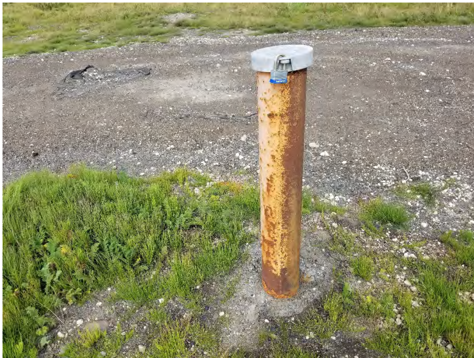
Ground Water Monitoring - Well DSA-MW-01 is secure and in good working condition.
