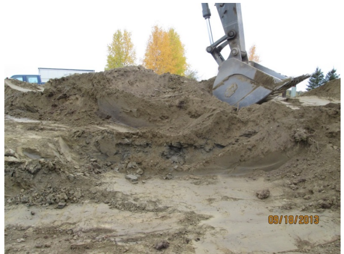
12) Dark gray silt with hydrocarbon odor in southwest portion of Excavation 1, facing south. September 18, 2013.
