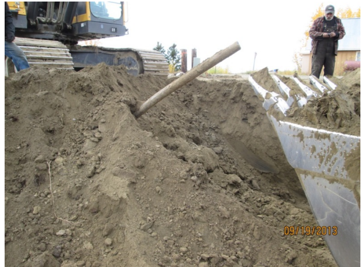
16) Another view of pipe in southwest corner of Excavation 1, facing west. September 19, 2013.
