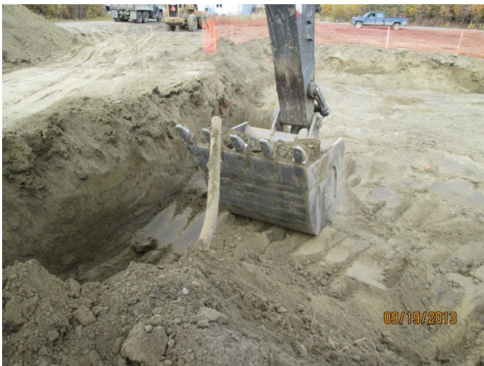
15) Another view of pipe in southwest corner of Excavation 1, facing north. September 19, 2013.
