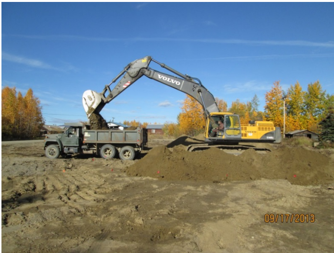
8) Loading contaminated soil from Excavation 1 into 10-cubic-yard dump truck for transport to the landfarm, facing north. September 17, 2013.
