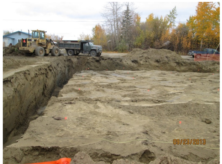
24) Western half of Excavation 2, facing north, showing area of dark-gray contaminated soil with strong hydrocarbon odor at northwest corner of excavation. September 23, 2013.
