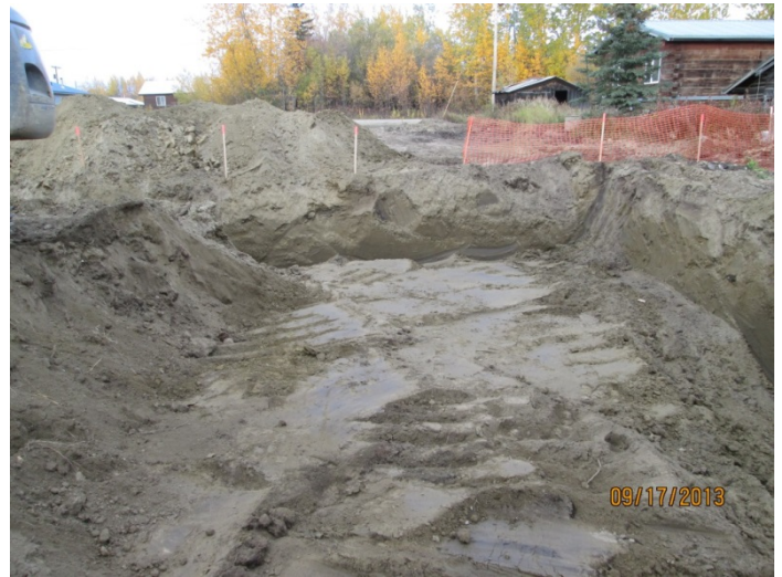
10) Northeast corner of Excavation 1 with deeper excavation for footer at perimeter, facing north. September 17, 2013.
