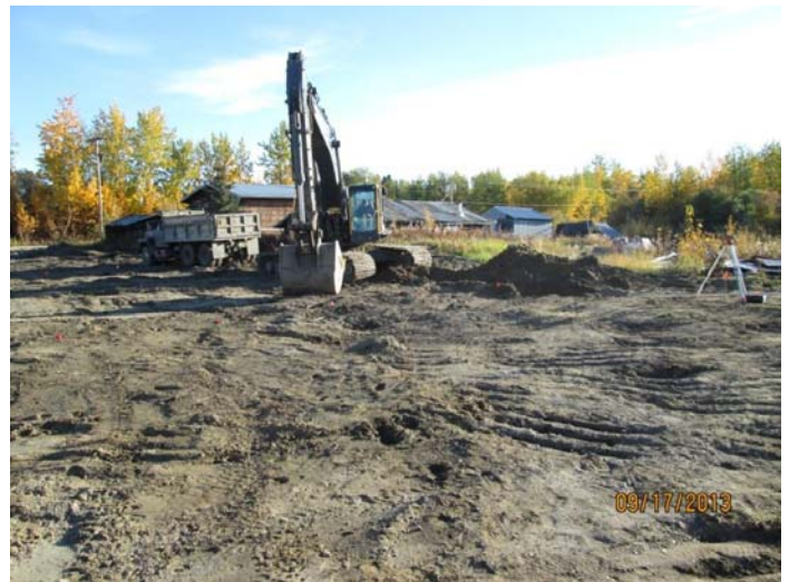
5) Starting to excavate at southeast corner of site, following grubbing. Facing northeast. September 17, 2013.
