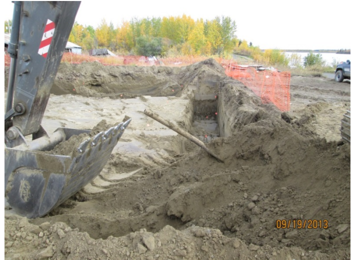
17) Another view of pipe in southwest corner of Excavation 1, facing east. September 19, 2013.
