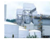
VIRGINIA CITY, VA, USA CFB scrubbers, PJFF and ESP Customer: Dominion Energy Capacity: 2 × 335 MWel, 2 × 1,046,000 acfm Fuel: Waste coal, biomass Start-up: 2011
