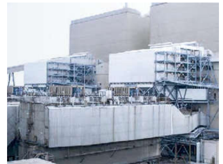
High-dust configuration at Hoosier Energy Merom Power Station, Units 1 & 2, Sullivan (IN), USA
