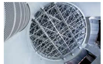
Scrubber at Neurath Power Plant, Germany
