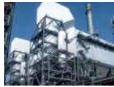
SANDOW, TEXAS COUNTY, USA Wet limestone FGD Customer: RWE Power Capacity: 2 × 1,100 MWel, 2 × 4,850,000 m 3 /h [stp, wet] Fuel: Lignite Start-up: 2011
